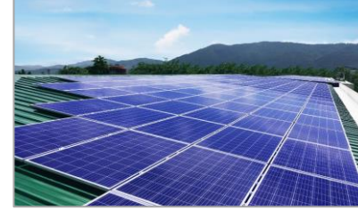
FEU Roosevelt Philippines 99 kWp, 2018
