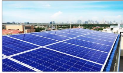
GPI Building Philippines 21.4 kWp , 2014
