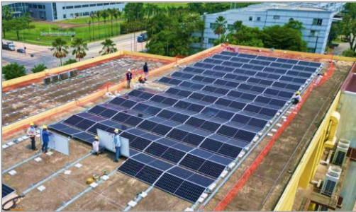
T&C Manufacturing, Singapore 423 kWp, October 2023
