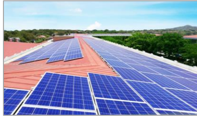
St Louis College Philippines 200 kWp, 2016
