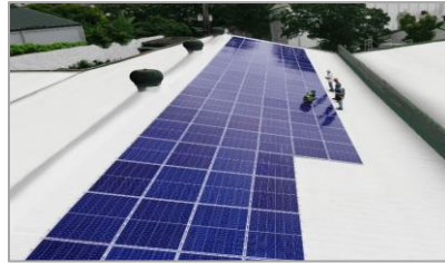
Baesa Warehouse Philippines 163 kWp, 2020
