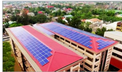
University of St. Louis Philippines 192 kWp, 2017
