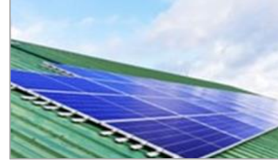
St Louis Maryheights Philippines 90 kWp, 2022
