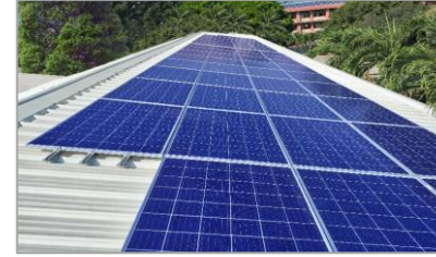
St Louis College –Cebu Philippines 172 kWp, 2018
