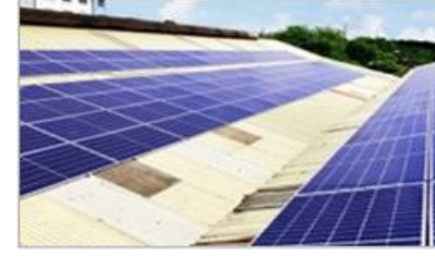
MD Juan Enterprises Philippines 72 kWp, 2022
