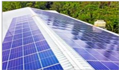
PrimeVibe Dressing Plant Philippines 143 kWp, 2022
